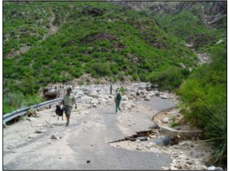
Damage to road from a debris flow in Sabino Canyon. (Photo from Arizona Geological Survey Open File Report 08-05)
